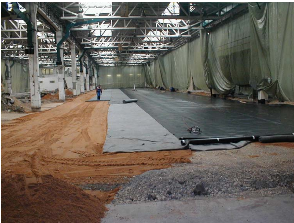
A plastic foil to prevent leaks of harmful substances to the underground is part of the floor structure used in manufacturing halls
